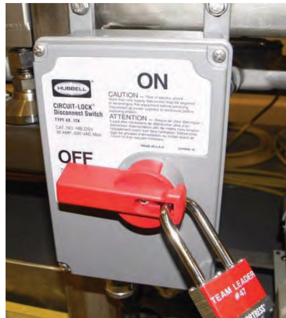
Figure 2-2: Typical Electrical Disconnect
