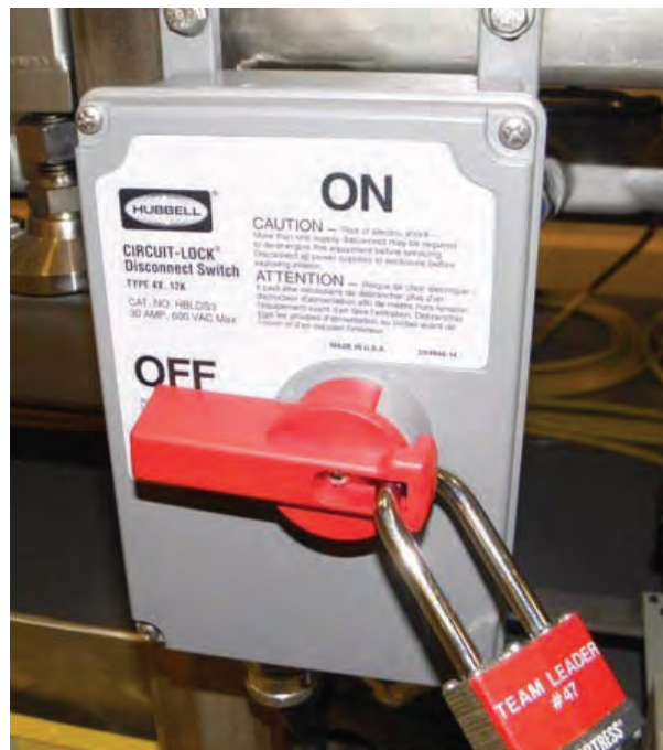
Figure 2-4: A typical electrical disconnect that is locked out in the OFF position
